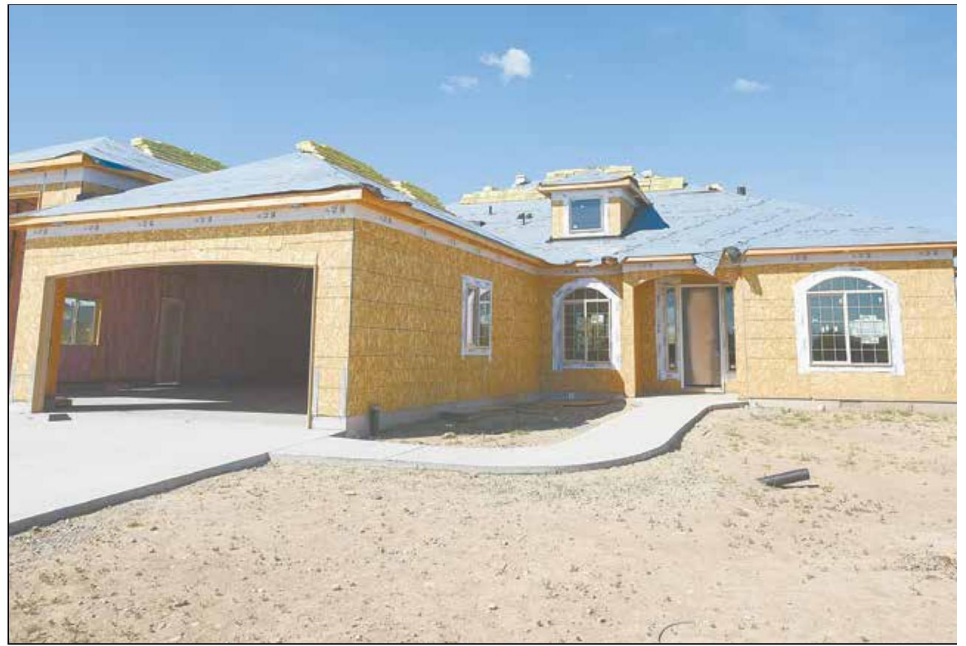
Roofing materials rest on the ceiling of a house under construction located on Morning Sky Avenue in Meridian on May 2, 2018
